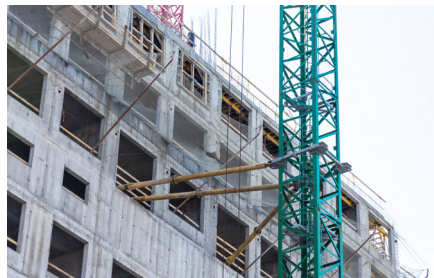
b) Tower crane support
