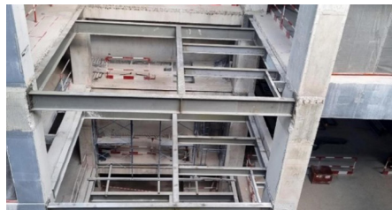
b) The steel frames are connected by anchors to the reinforced concrete structure
