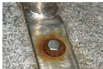
b) Heavy corrosion of a zinc plated carbon-steel washer
