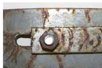
c) Corrosion of a steel bracket in an indoor swimming pool
